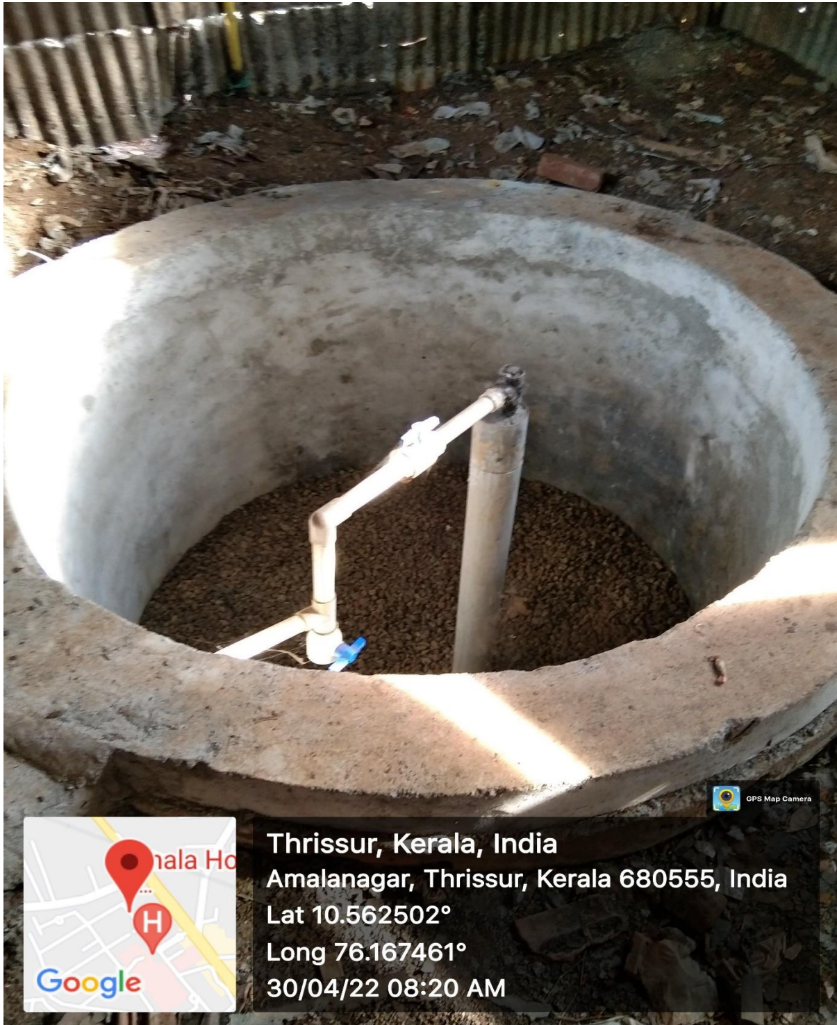
ACON, BIOGAS PLANT, LEFT SIDE OF THE COLLEGE BUILDING
