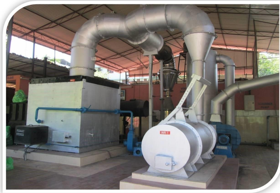
ACON, INCINERATOR, WASTE TREATMENT PLANT
