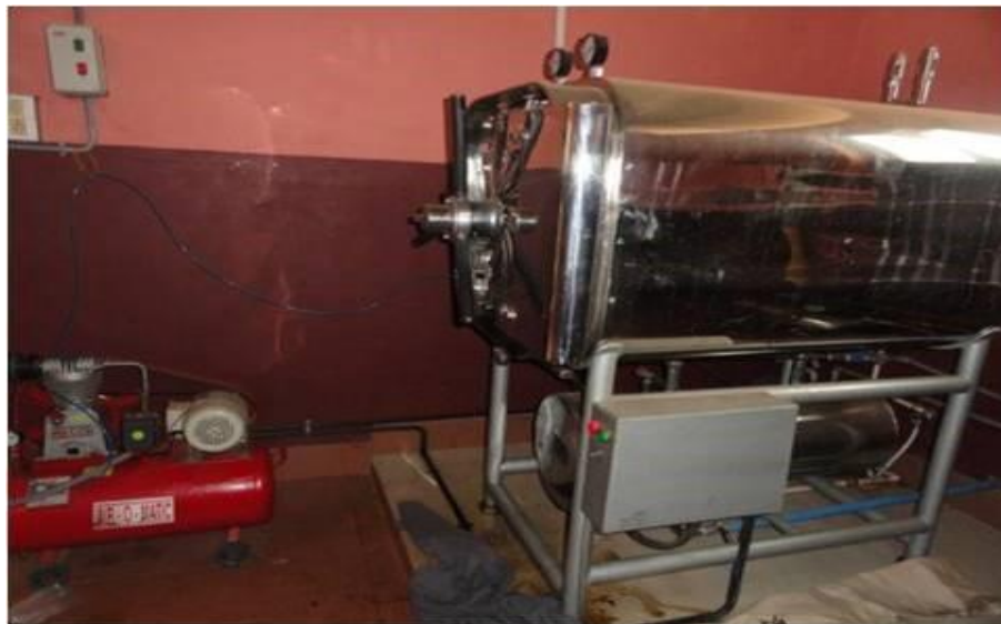
ACON, AUTOCLAVE, WASTE TREATMENT PLANT
