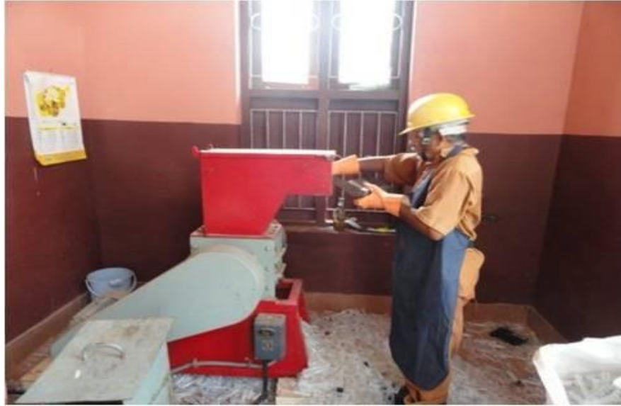
ACON, INCINERATOR, WASTE TREATMENT PLANT
