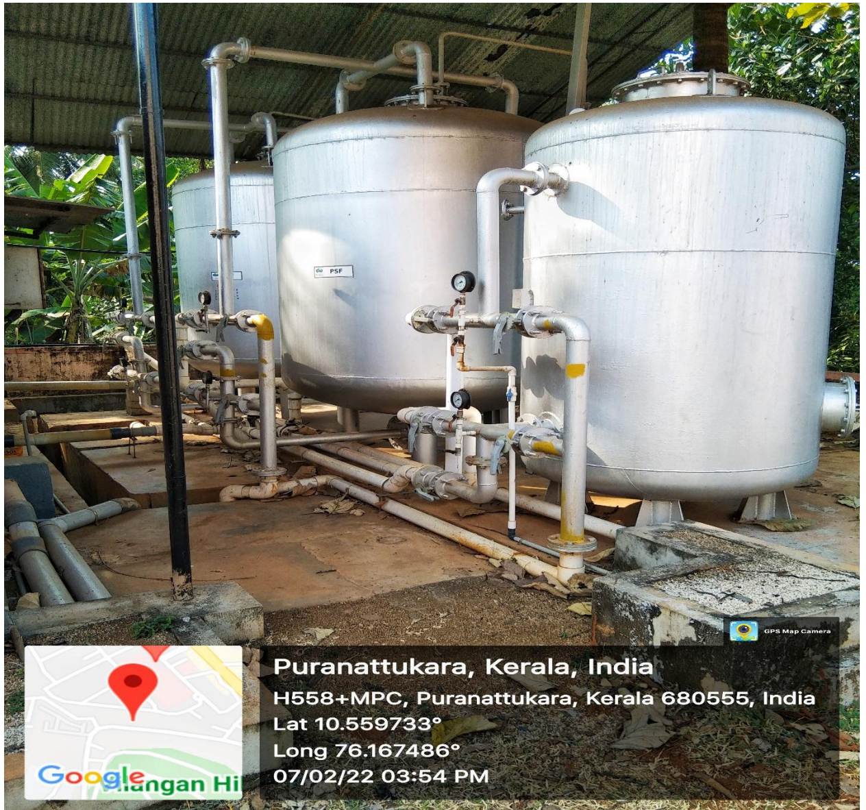
ACON, FILTER FEED TANK, WATER TREATMENT PLANT
