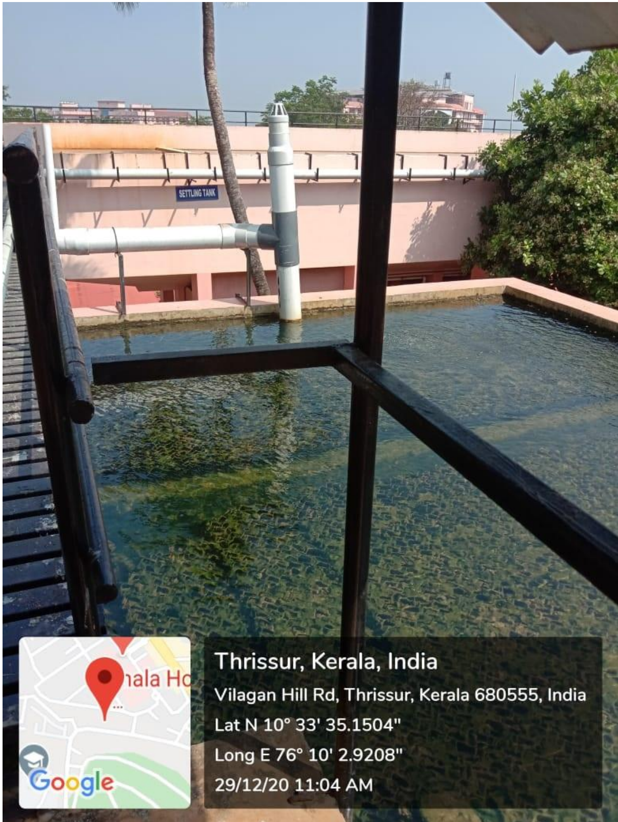
ACON, SETTLING TANK, WASTE WATER RECYCLING PLANT
